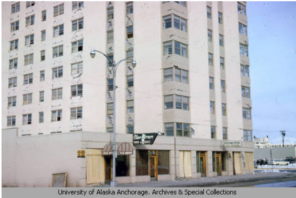
Figure 10. Damage to the McKinley Tower (Mount McKinley Building at the time of the earthquake), Anchorage, Alaska, 1964. Compare the x-shaped cracks below the windows with those on the Inlet Tower (Stop 19). (Photograph from Judith and Malcolm McDonald papers, Archives and Special Collections, Consortium Library, University of Alaska Anchorage ID uaa-hmc-0619-s2-f22-20.)
