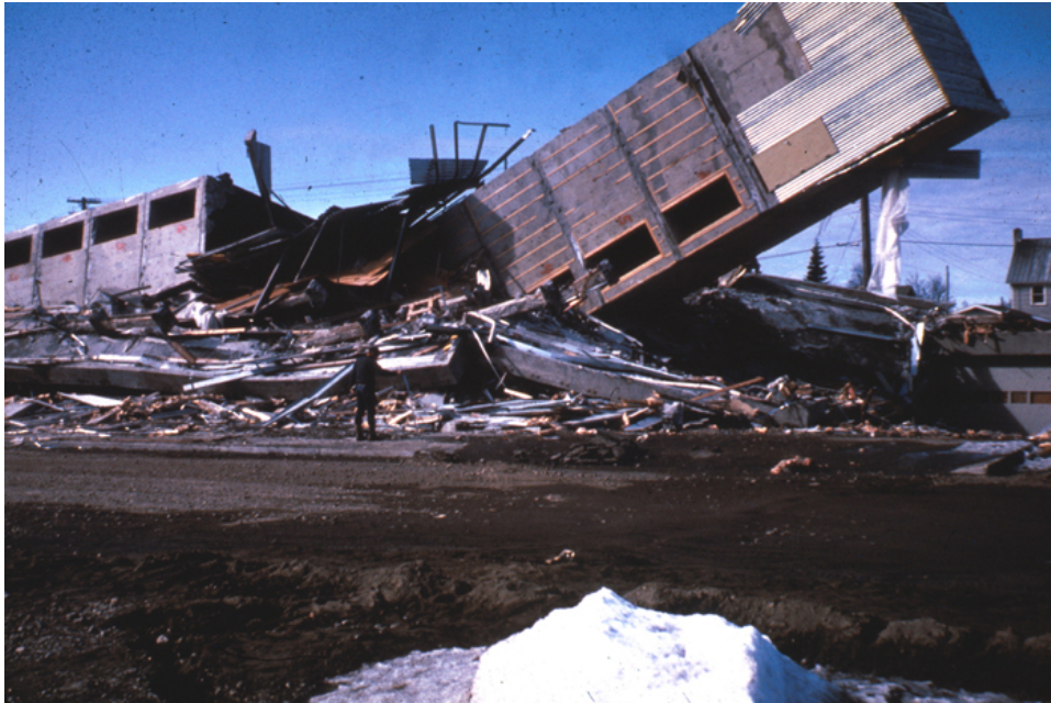
Figure 33. The remains of the Four Seasons Apartment Building, Anchorage, Alaska, 1964. The tilted column on the right was the combined elevator shaft and stairwell. (Photograph from U.S. Geological Survey Photographic Library, ID aeq00026.)
